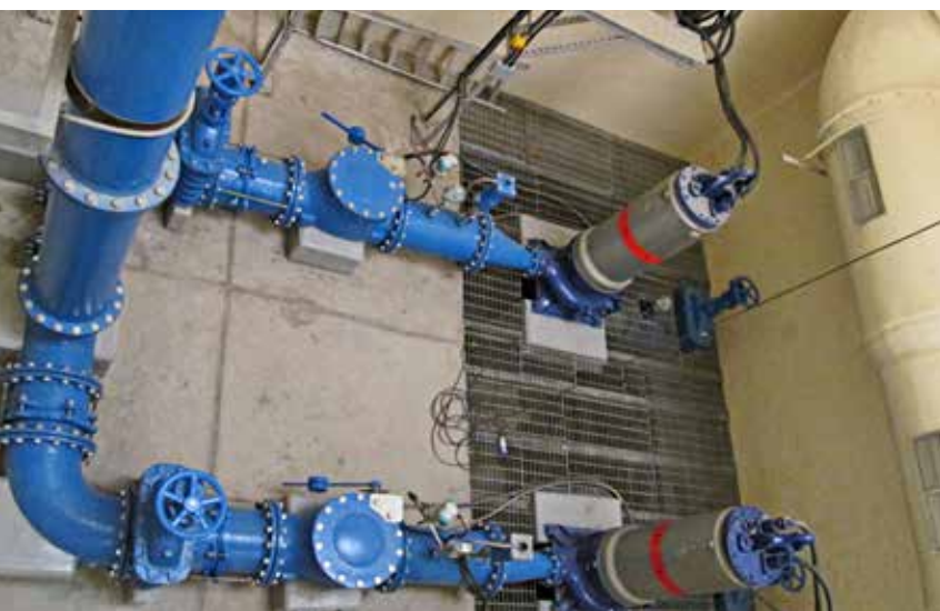
Stations de pompage, Abu Dhabi, EAU
